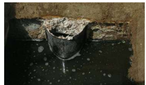
Illustration 1 - Concrete Corrosion Around Outlet Baffle
