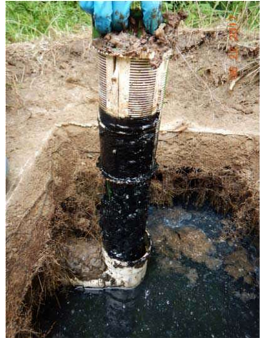
Illustration 2 – Clogged Effluent Filter
